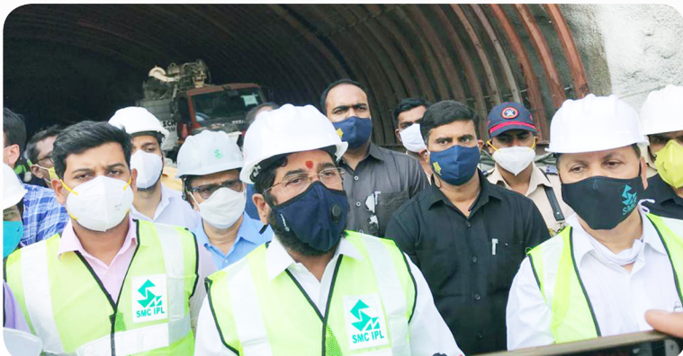
Airoli Katai Naka Tunnel, inaugural blast by Shri Eknath Shinde, UD Minister for Government of Maharashtra
